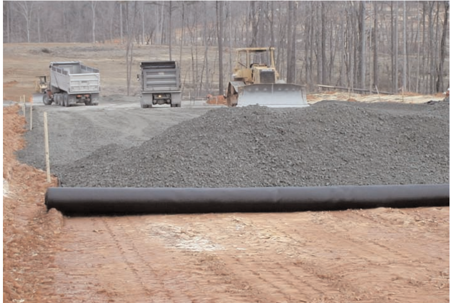
A well graded aggregate base course (ABC) was placed directly over the geosynthetic.
