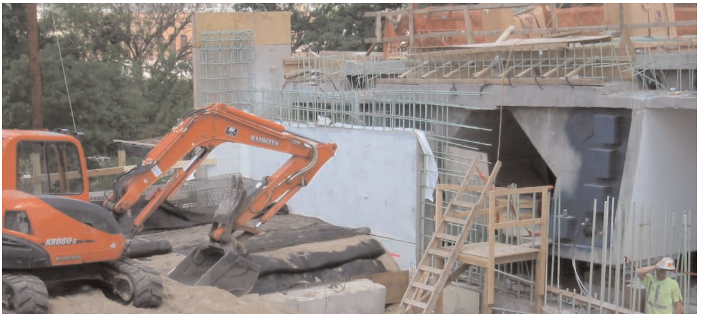
Temporary fabric wrapped wall at bridge abutment will allow Gabion retaining wall and bridge to be built concurrently.
