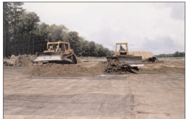
The installed cost of the geogrid test section was 46% more than the installation cost of the Geolon® geotextile.
