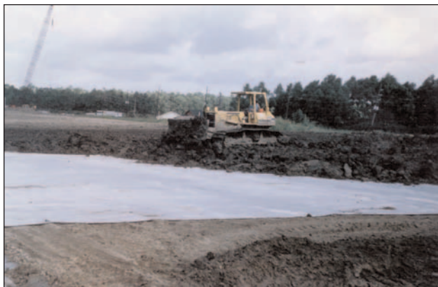
Though both the geogrid and geotextiles performed as expected, the geotextile is the logical choice for this application.
