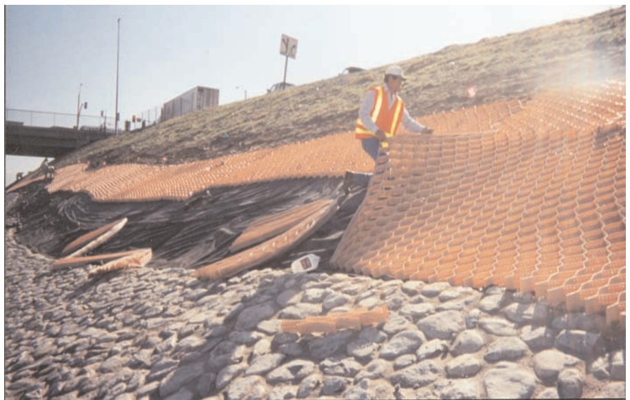
After the slope is graded, Filterweave® woven geotextile is placed. Micraweb® is expanded over the Filterweave®
