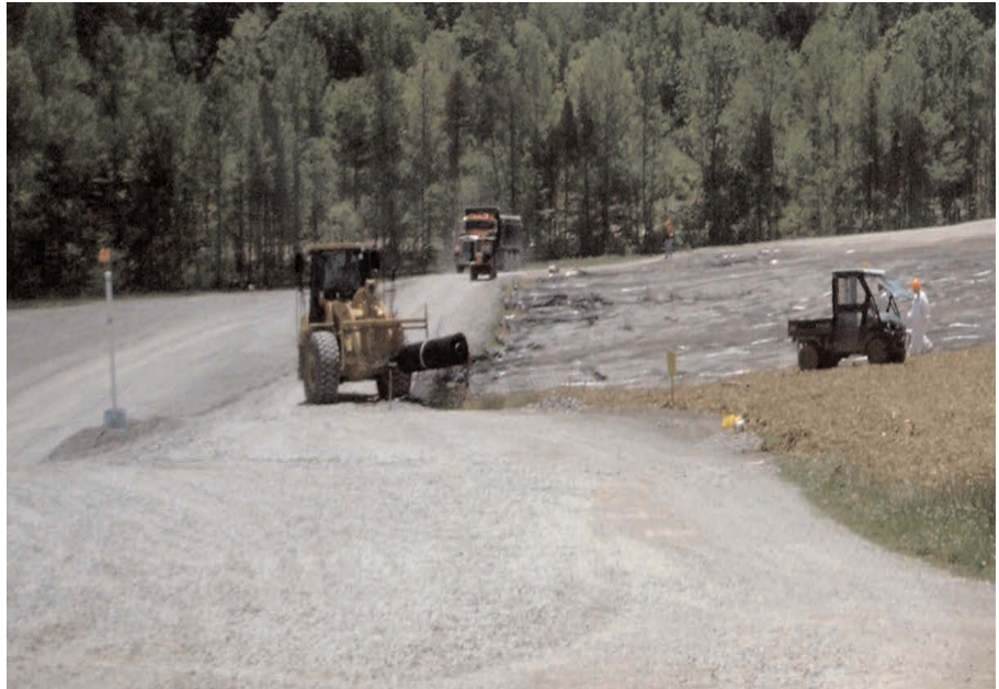
Miragrid® 20XT was installed using an off-road vehicle to pull the geogrid over the cap.
