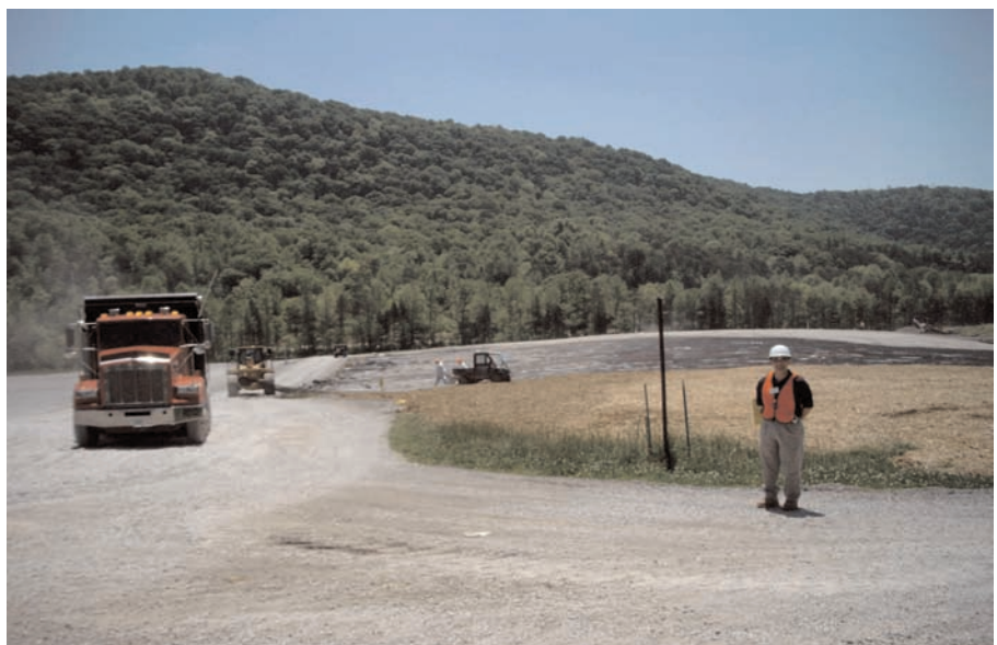
1.1 million square feet of Miragrid® 20XT is being installed throughout the site.
