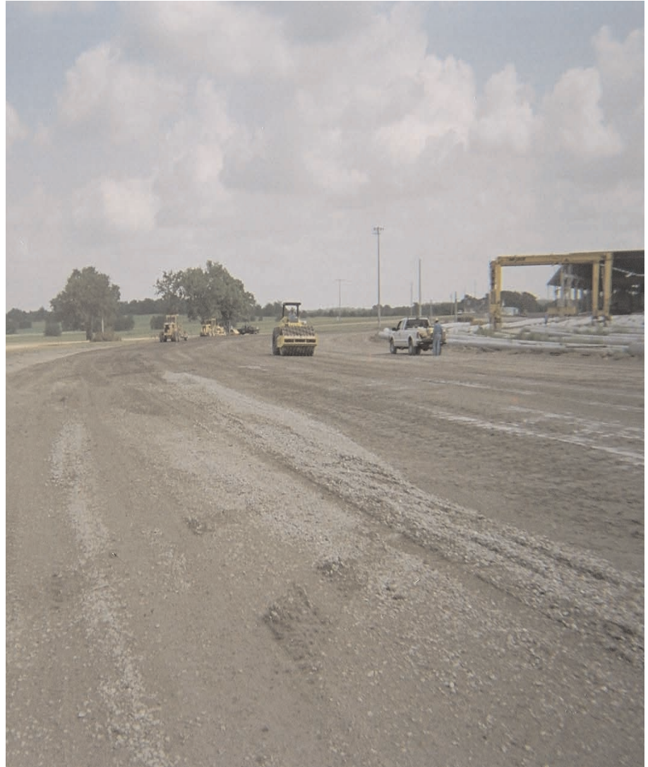
Newly constructed gantry crane wheel path area where Mirafi® HP770 was installed.
