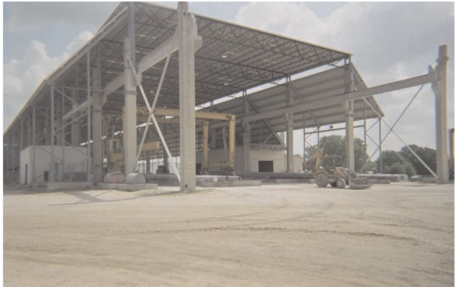
Pre-cast plant with gantry crane inside.
