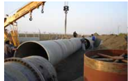
1.4m \phi pipes for effluent disposal
