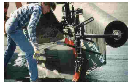
Figure 3: The Polyfelt PGM paving fabric was installed using a laying device fixed to the bucket of a front end loader. Brushes behind the fabric ensure smooth laying.
