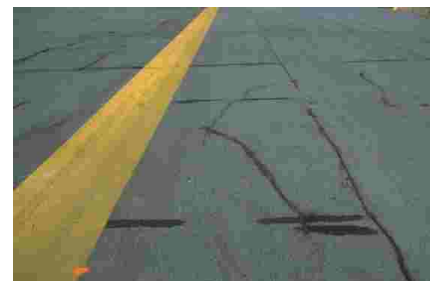
Figure 2: Reflection cracks from the old concrete surface
