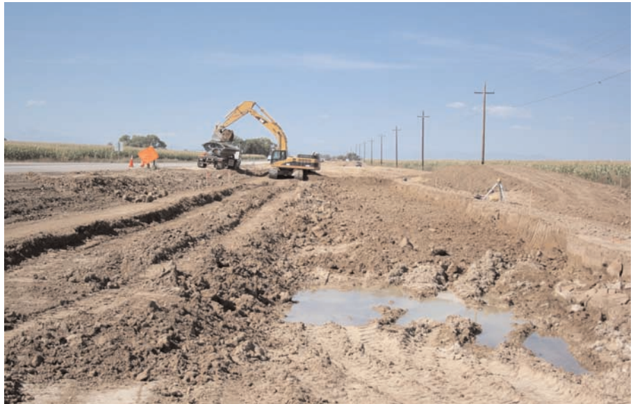
Condition of existing roadway after the section was torn out.
