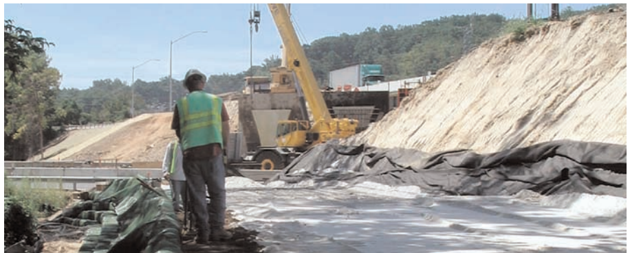
Below: Compaction of soil at the face of the slope for vegetation.
