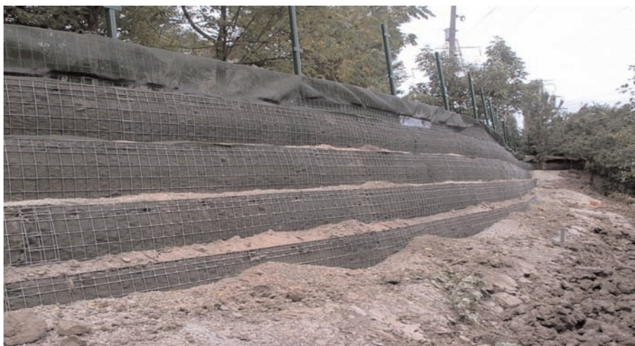
Miramesh® GR is selected as the face wrap to protect the vegetation from erosion.
