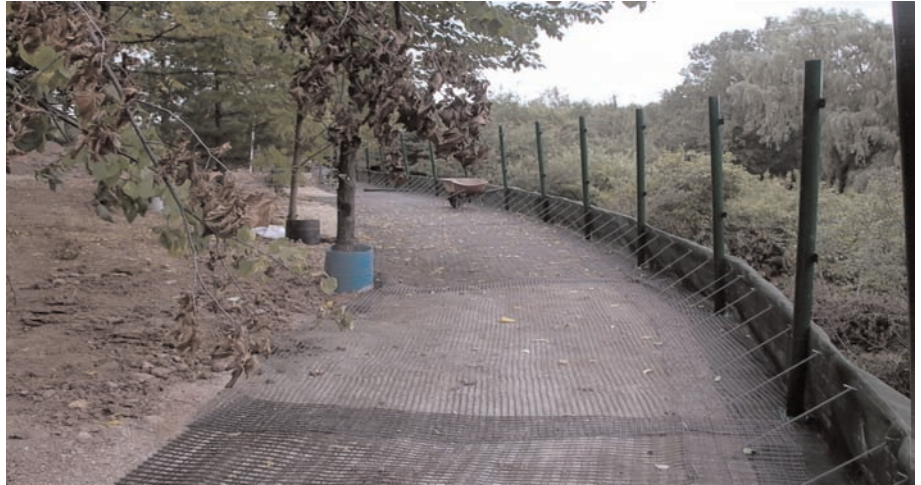
Each basket overlapped 100mm (4in.) Miragrid® 3XT was placed to the front face, then Miramesh® GR was installed along the wire struts.
