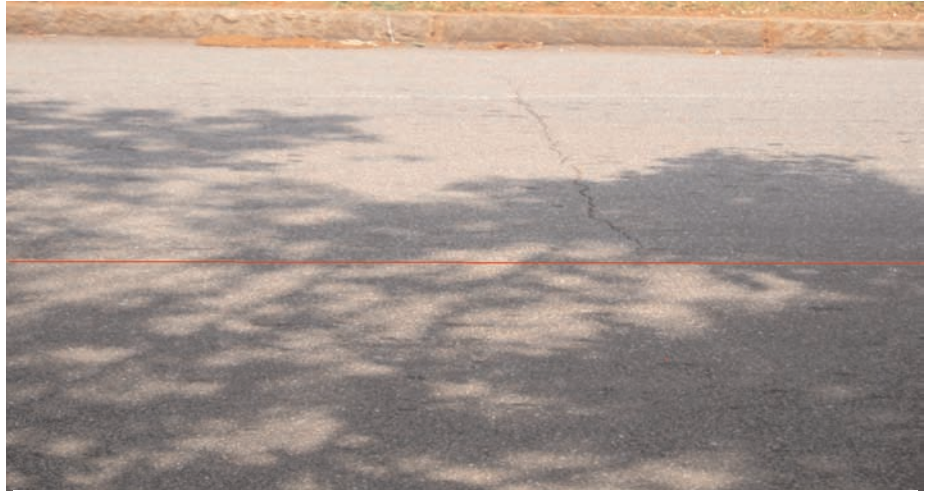
After 5 years: Top half of photo shows the control section with longitudinal cracking. The bottom half, with no cracks, is the Mirafi® FGC Pave Grid 50 test section.
