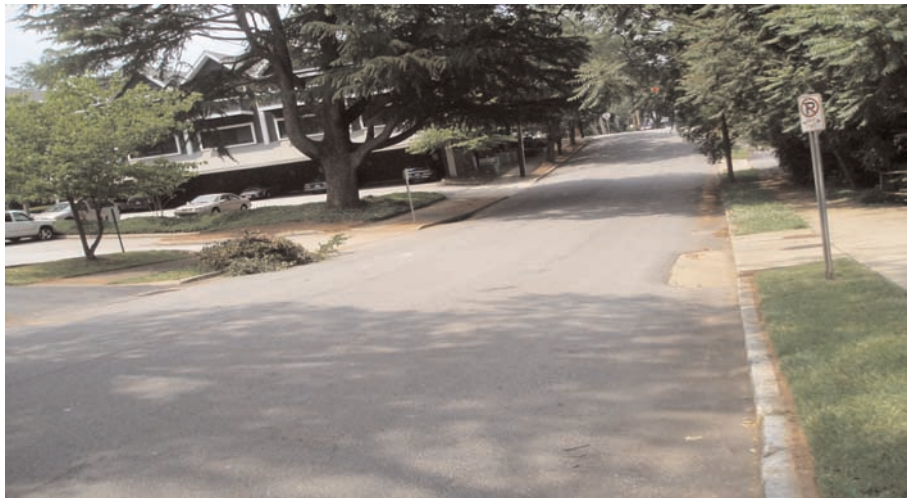
Evaluation of the Boyce Street trial proved paving grid composites can significantly delay reflective cracking.
