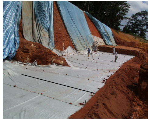
Fig. 6(a) 'Intelligent' geosynthetic placed in the structure as part of the soil reinforcement system
