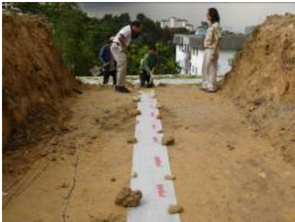
Fig.7 Trench excavated at the top of slope for placement of the geosynthetic to monitor movements of existing slope
