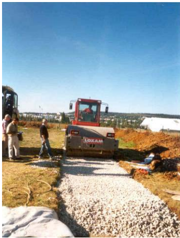
Figure 5(a). Damage test September 2002.
