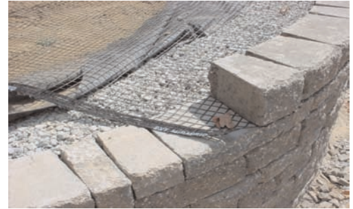
Lower retaining wall construction: Miragrid® 2XT and nonwoven filtration and drainage geotextile.
