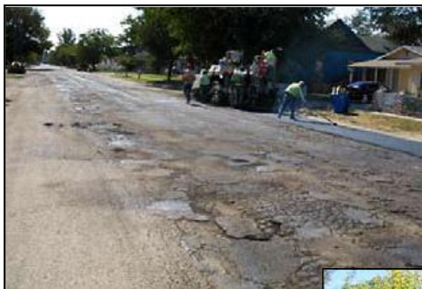
Figure 1. Limited areas of sheet patching and distressed pavement before fabric placement.
