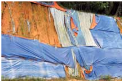
Conventional tarpaulins deteriorate quickly under UV exposure
