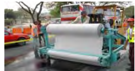
Laying of Polyfelt® PGM14 on tack coat with a paving installation rig.
