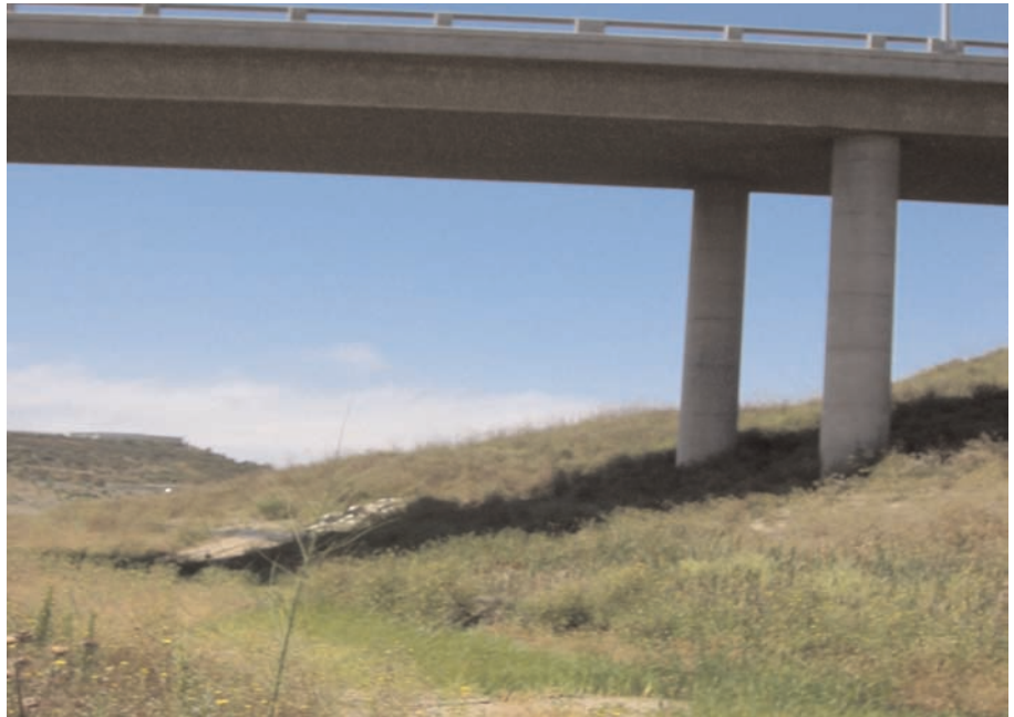
This environmentally sensitive area in the Talega community is now hydraulically sound and promotes habitat restoration.
