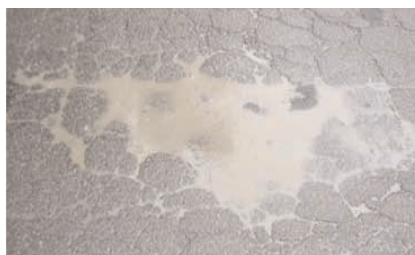
Asphalt showing fatigued pavement surface
