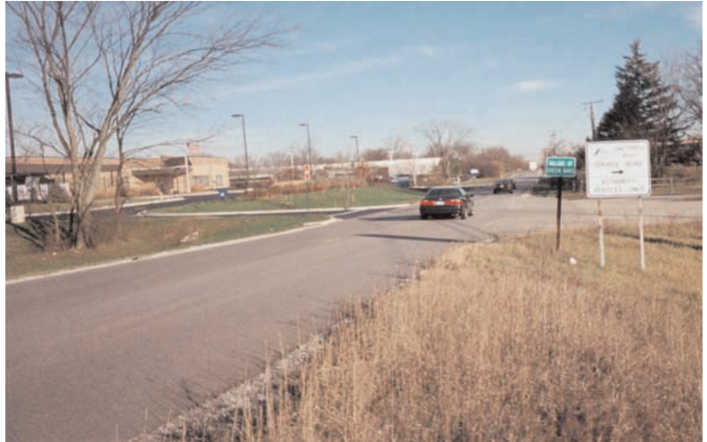
The completed Bradley Road project maintained its integrity throughout a harsh winter season with considerable freeze cycles.
