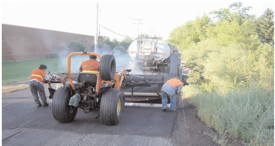
Mirafi® MPV700 was installed, and a polymer asphalt binder was used in this installation.
