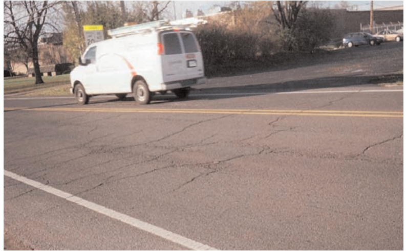
Older roads within the area that lack paving fabrics suffered from unnecessary cracking and deterioration.
