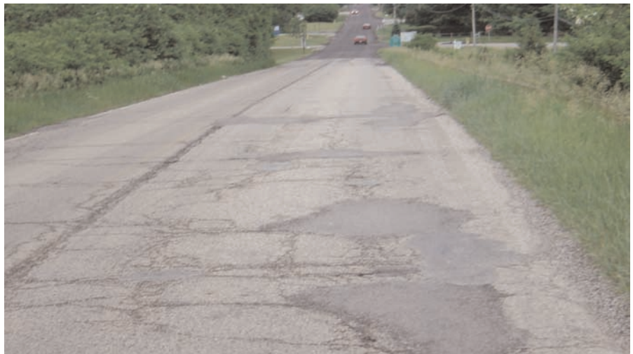
Bradley road was in dire need of restoration. Mirafi® MPV700 was chosen as the economical solution.
