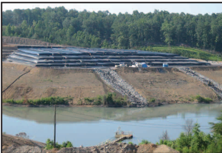
One 4-layer stack of Geotube® containers was buried before another four layers were placed and filled on top.
