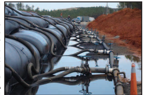
A manifold system was used to control the flow between the Geotube® units.
