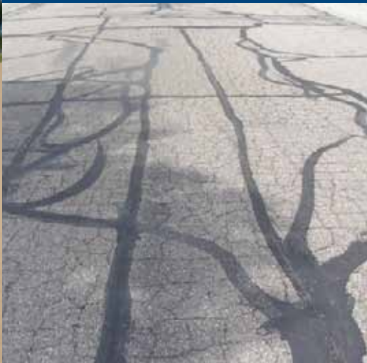
FILL MAJOR CRACKS
