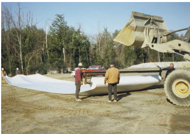
The contractor fabricated a lifting beam and spindle attachment to install the HS4200.
