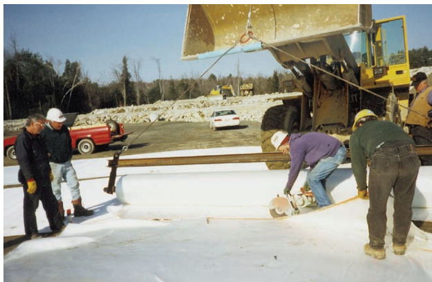
Geolon® HS4200 master rolls were delivered to the job site for efficient coverage.
