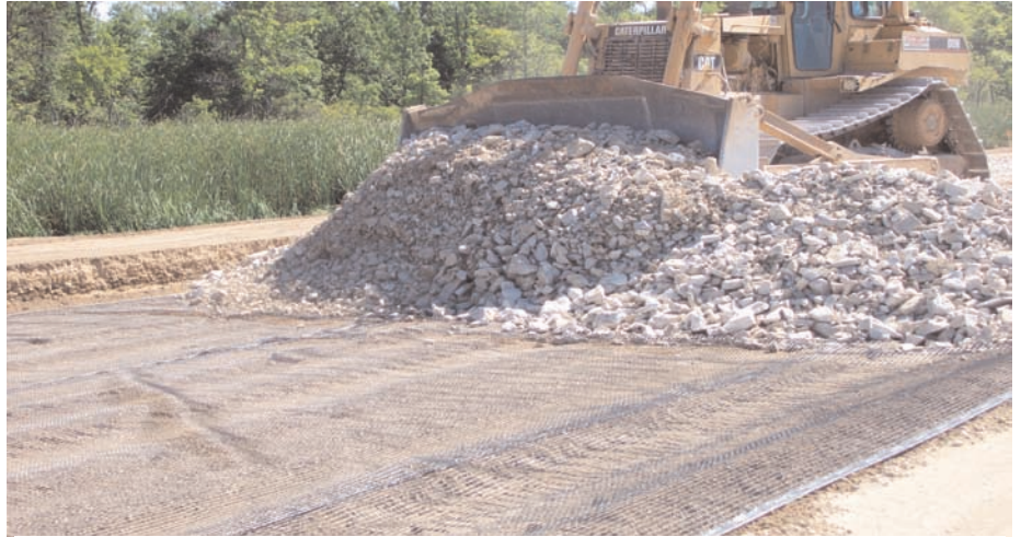
Sixteen inches of breaker rock was placed and compacted over the Mirafi® BXG11 followed by 12in of crushed aggregate.
