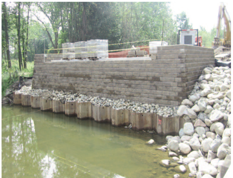
Block facade is placed as geotextile reinforcement and stone lifts are brought up.
