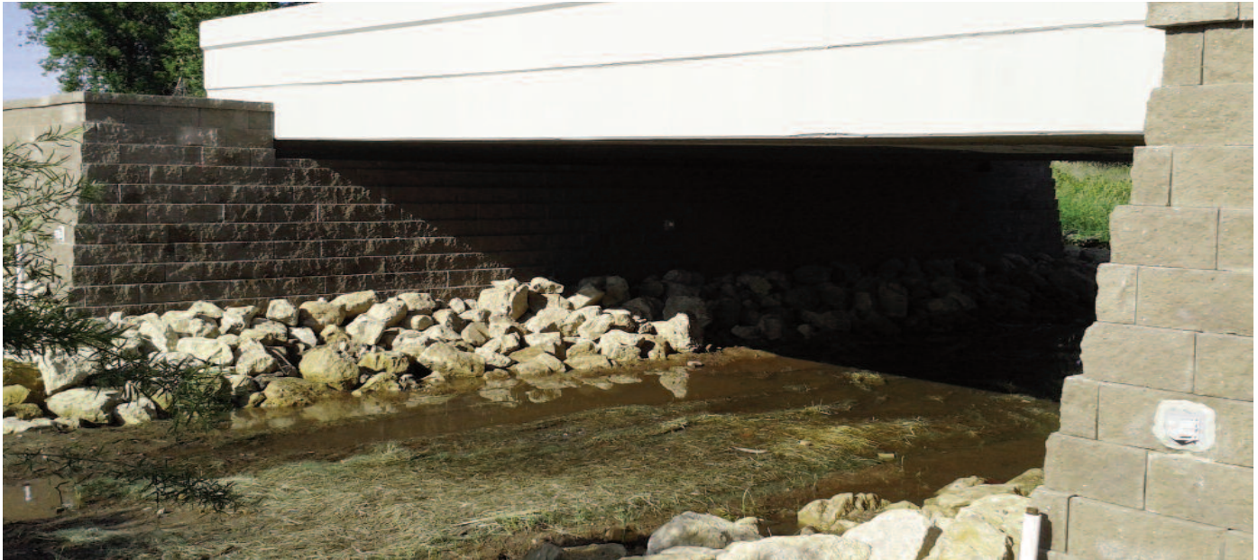
The completed project with both abutments and the roadway placed and ready for traffic.
