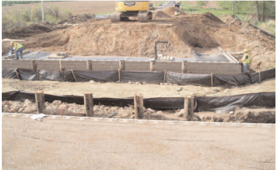
Overview of the project site after the first courses of block were installed
