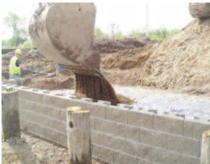
Backfilling behind the precast block. The geotextile, block, and aggregate work together to form a reinforced earth system.
