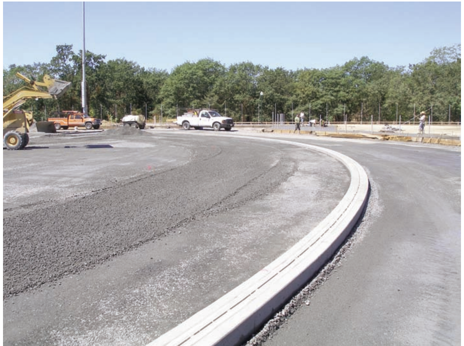
Cutting and placing the fabric for curves around the perimeter was simple and quick.
