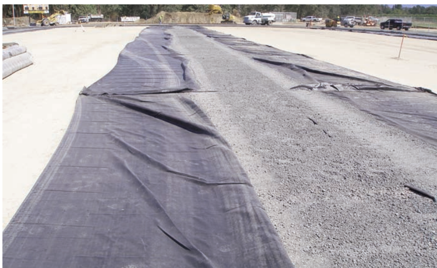
Mirafi® HP270 was deployed as a drainage fabric under the entire field as well as for separation and reinforcement below grade.
