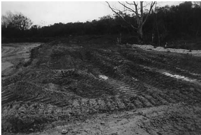
Weak subgrade not suitable for construction
