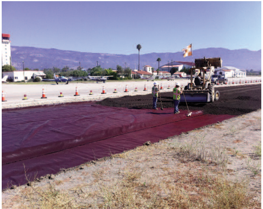
Workers help spread the asphalt grindings evenly over Mirafi® RS380i high strength geotextile.
