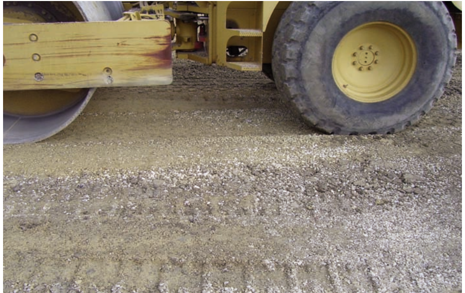
Proof roll showing some rutting of subgrade prior to placement of Mirafi® RS380i
