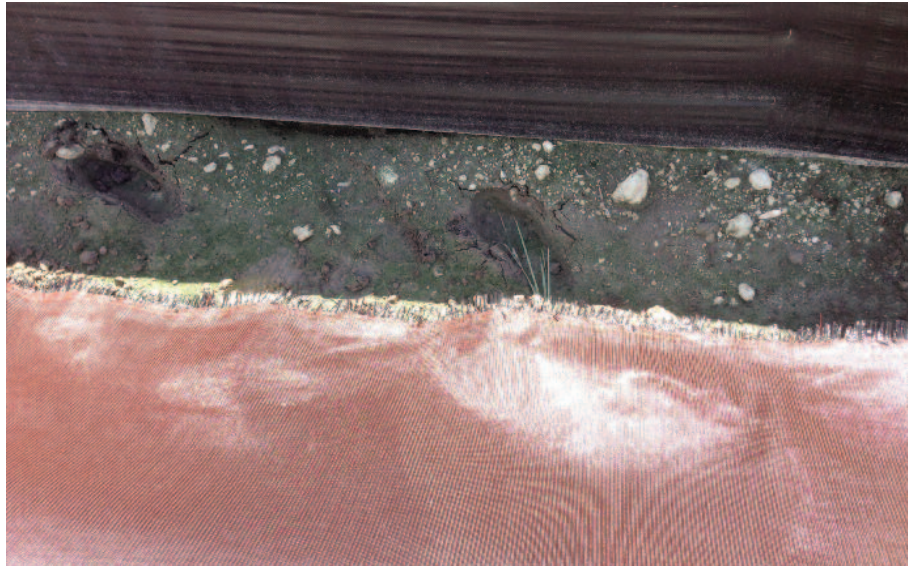
Condition of the soft Dredge spoils subgrade at time of construction.
