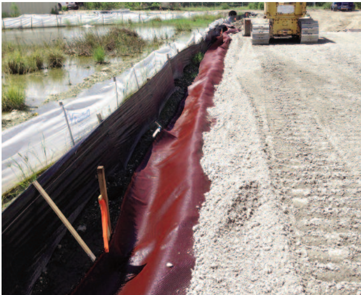
Leveling the compacted lift of Limerock Base aggregate on Mirafi® RS580i before placing Mirafi® BXG12. Finished flexible pavement surface.
