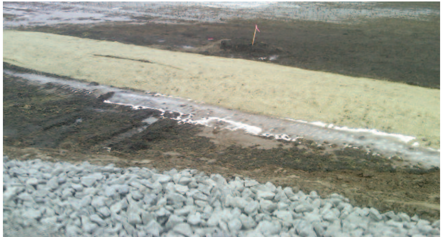
The project site had saturated soils with very poor bearing capacity.
