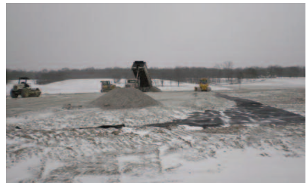
Mirafi® HP570 is placed and aggregate is being pushed out and compacted.
