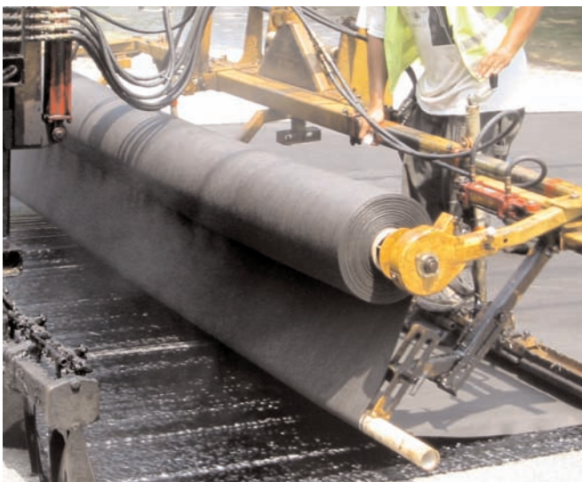
After the asphalt cement was applied to the existing pavement, Mirafi® MPV500 was installed.
