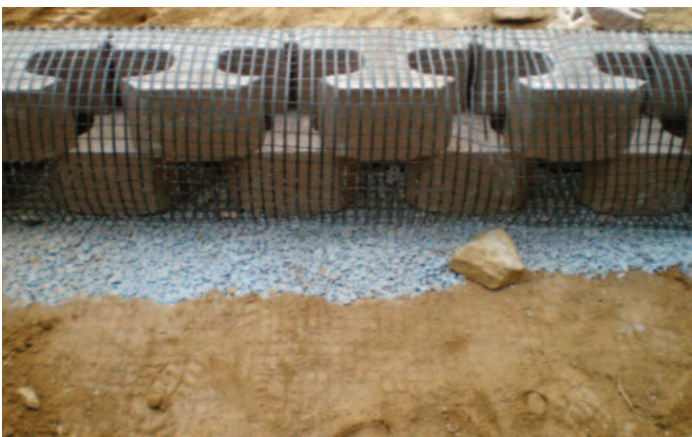
Geogrid draped over the blocks while backfill and aggregate drainage liner is placed.
