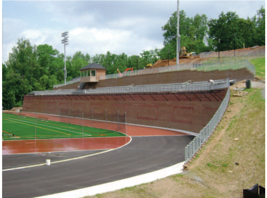
A two tier retaining wall allows for proper grading and placement of the stadium seating.
