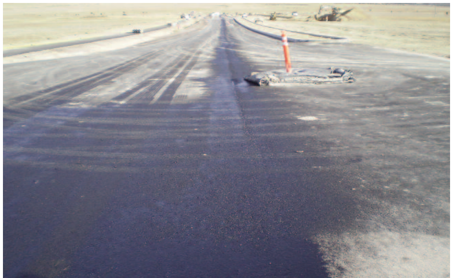
Final lift of asphalt will be placed before open to final service.
