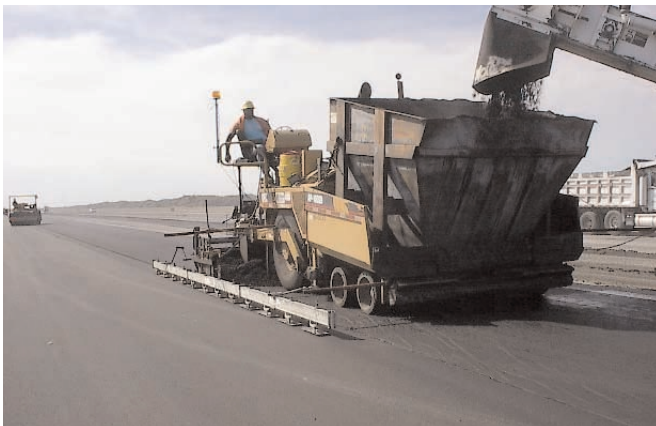
Screed machine spreading hot asphalt over Mirafi® MPV 400. This automated machine levels the asphalt to the correct height.
