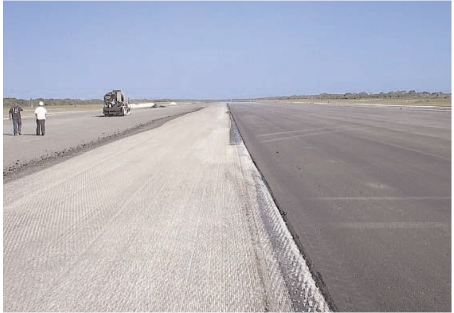
Above: The milled surface on the left, and the binder, right, 1.5" with 20% recycled asphalt.
