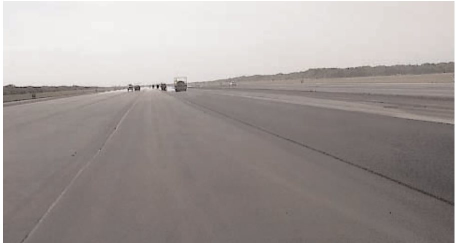
A paving fabric was chosen to prevent the degradation of the pavement.
