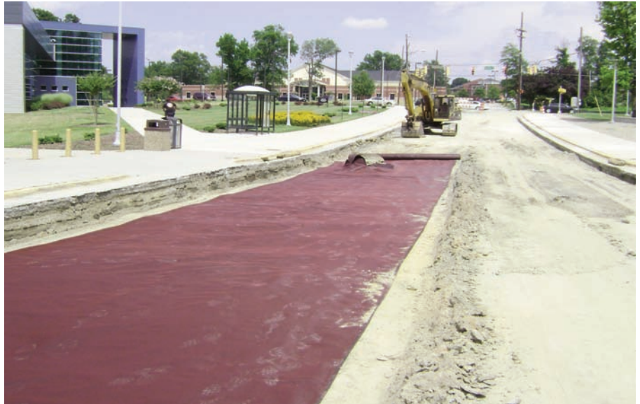
Mirafi® RS580i is placed on the subgrade 9" below the required base course elevation. Rutting of the subgrade material due to the construction traffic can be seen at the right side of the photo.
