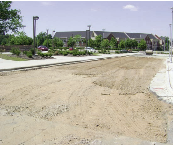
Base course finished elevation before the final compaction was completed prior to asphalt being placed.
