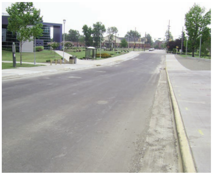
Roadway shown with asphalt base material installed prior to the final asphalt wear surface being placed.
