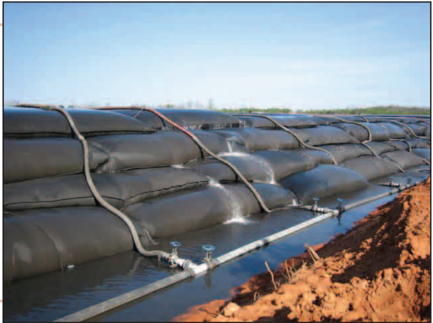
Geotube® Containment and Dewatering technology was used to dispose of slurry waste from North River Mine.
