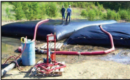
To prove the efficiency of Geotube® dewatering, a full scale trial was performed.
