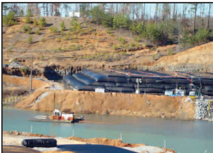
A dredge pumped slurry waste from the lagoon to the Geotube® containers.
