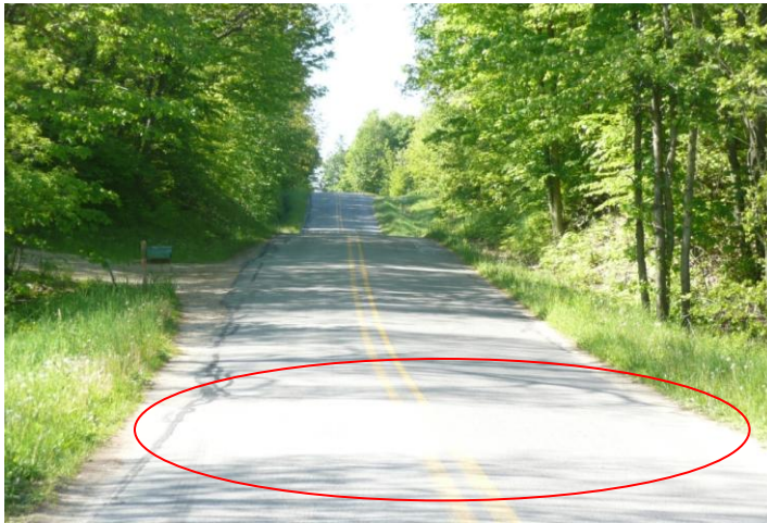
23 Photograph 4. Van Buren County Test Section 24 Fabric delaminated due to subsurface water pressure
